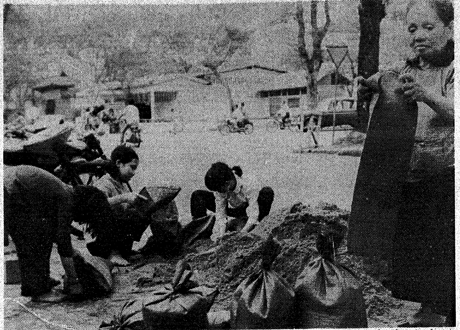
All members of a Chinese family turn out in closed their laundry shop for the day to devote downtown Saigon to construct a bunker. They all efforts to the task. (AP Radiophoto)
